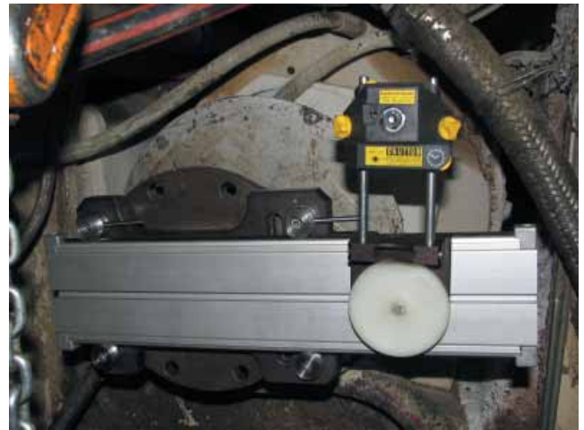
Figure 3: The specially designed cardan shaft bracket. The assembly allows the laser & receiver to be mounted with an offset to each other.
