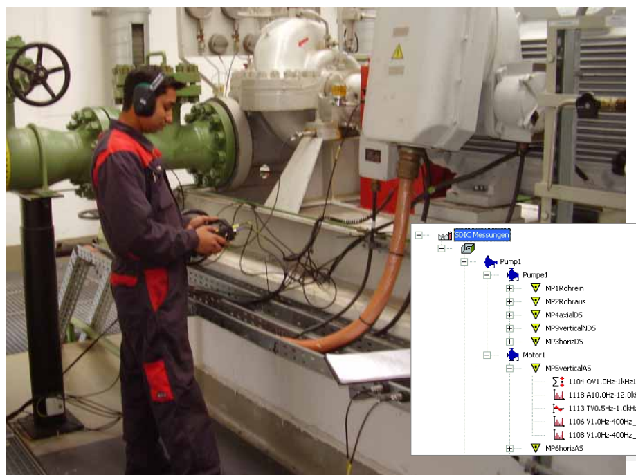
Fig. 1: Vibration measurement on a pump
